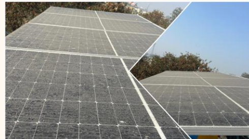
Solar Energy System
